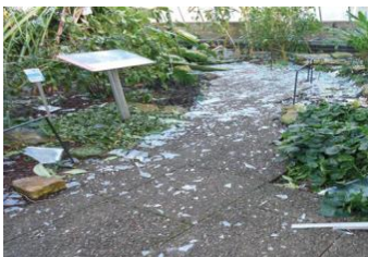
Storm damage has resulted in multiple broken panes of glass in the glasshouses at Inverleith in Edinburgh, leaving tender plants exposed to the elements.
